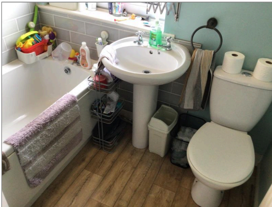
Photo - 8 Bathroom fittings
